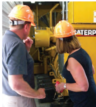
Steve Foss, Manager, gives Emerson a tour of LJEC's peak shaving generator.
