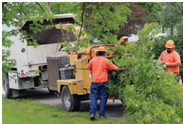
LJEC's tree crew has spent the last 15 years clearing up to 100 miles of line per year.
