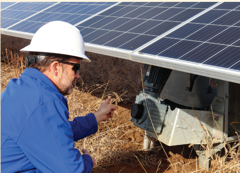
Energy Use Coordinator Matt Lambert inspects the mechanism under a solar panel. Lambert is FreeState's main point of contact for solar or renewable information. He works directly with members on solar projects and is heavily involved with the cooperative's five solar sites, providing insight and education about project benefits.
