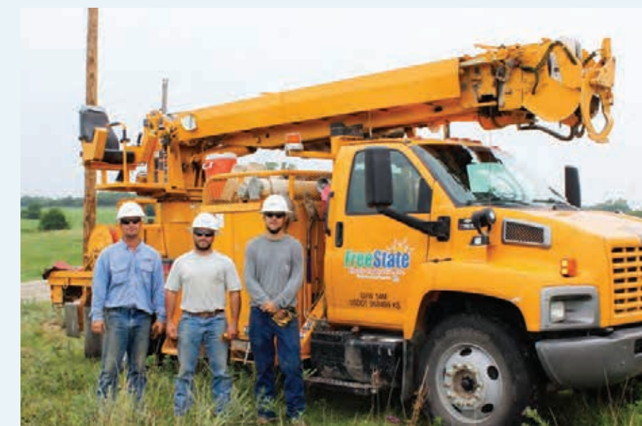
From left: Bryce Best, Journeyman Lineman, Noah Schreck, Journeyman Lineman Apprentice 3, and Brooks Vaughn Journeyman Lineman Crew Foreman, set polls for new service.
