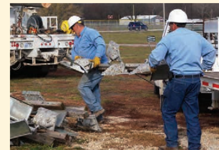
Linemen Bill Likes (left) and Rick Smoots remove poles that were damaged in a tornado at the Leavenworth County Fairgrounds—a community service project initiated by Smoots in 2010. The poles suffered damage when a tornado passed through town. Over the years, the condition of the poles had worsened and posed a safety issue for fairgrounds visitors.
