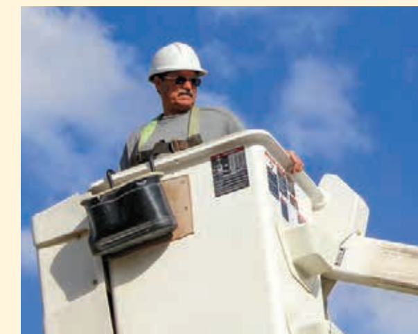
On May 31, 2017, FreeState Electric celebrated Rick Smoots' upcoming retirement after 50 years of dedicated service as a Lineman. Here he is working from one of FreeState's bucket trucks and is restoring power to members of the cooperative after an outage.
